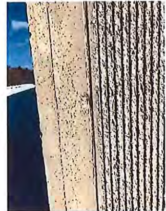
Aged Joint Sealant
