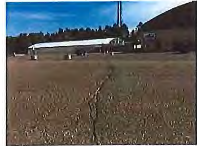
Cracked Parking Lot Pavement
