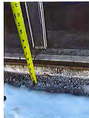
Trip Hazard at Main Entry
