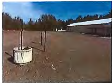
Cracked Parking Lot Pavement
