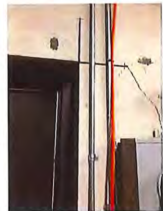
Overcut Door Openings
