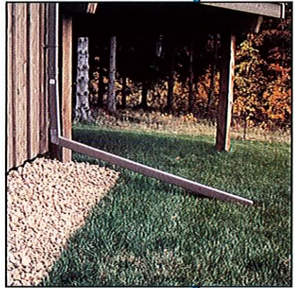
Directing your downspouts out into your yard helps keep your basement dry and reduces the inflow from your home.
