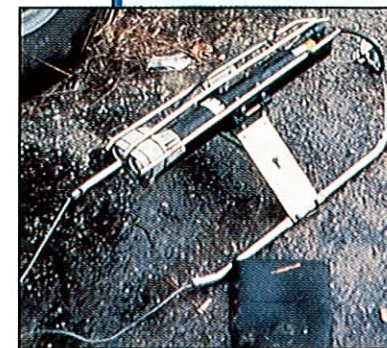
Inspecting sewer pipe with special video cameras helps WLSSD and cities locate leaks inexpensively without digging.
