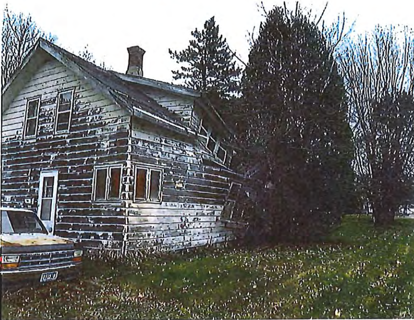
South dormer beginning to collapse due to failed supporting structure
