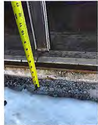
Trip Hazard at Main Entry
