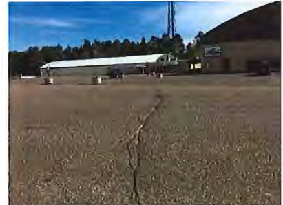
Cracked Parking Lot Pavement
