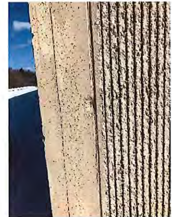
Aged Joint Sealant
