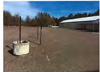
Cracked Parking Lot Pavement
