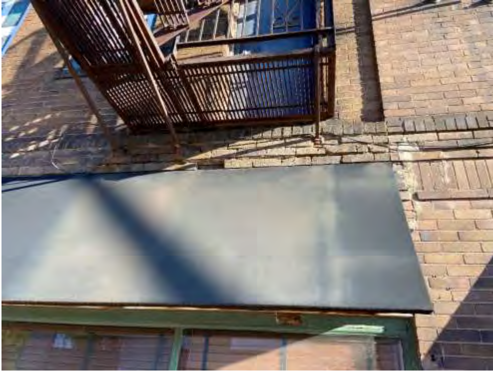
Photo 7: Brick Damage and Lower Connections
